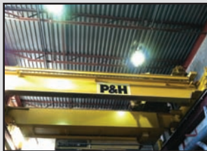
P & H BRIDGE CRANE
